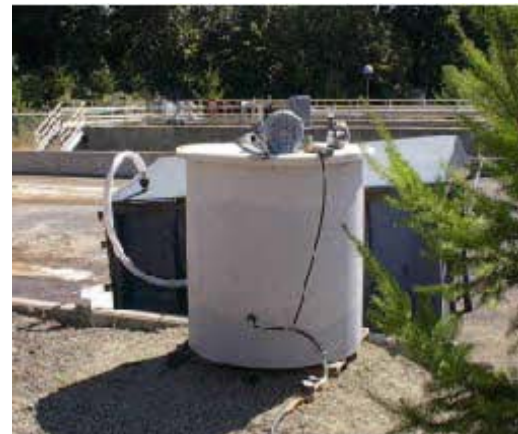
Wastewater Treatment Plant, Odour Control
